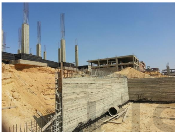
Fig. 2.(b). error in execution (non-retaining the adjacent Neighbour structures)
