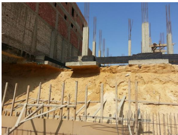
Fig. 2.(a). error in execution (non-retaining the adjacent Neighbour structures)
